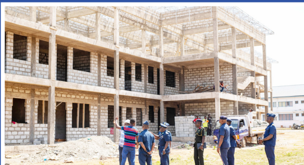
CAS INSPECTING THE CONSTRUCTION OF A 24-UNIT STUDIO ACCOMMODATION FOR AIRMEN AT THE AIR FORCE BASE, ACCRA.
