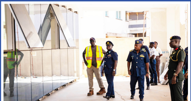
CAS INSPECTING THE PROGRESS OF WORK ON THE WOs AND SNCOs MESS AT THE AIR FORCE BASE, ACCRA.
